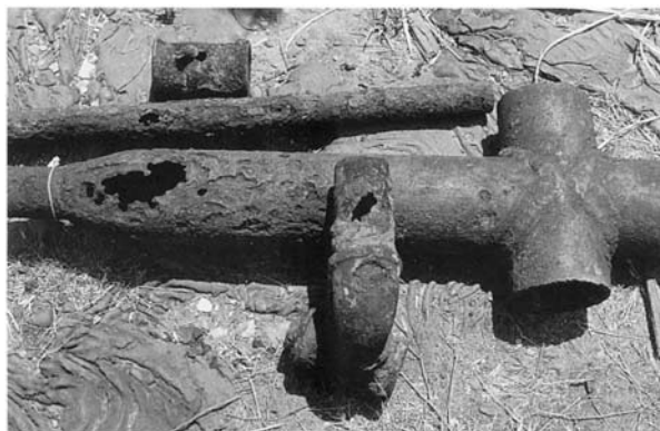
Corrosion of buried pipe.
